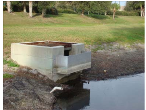
White PVC pipe exposed as it enters Lake 1-7. The pipe is blocked somewhere between this entrance point and the valve shown above. The underground length of the pipe is approximately 100 yards.
