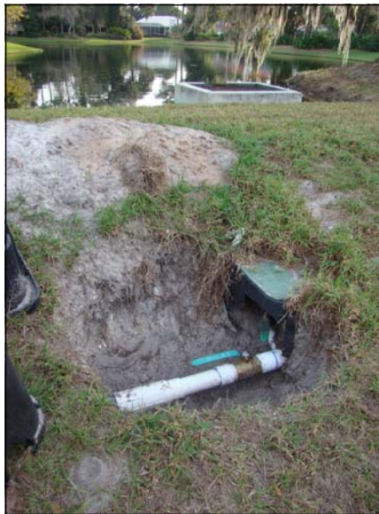
New Valve Installed near Lake 1-7 (in background) controls supplemental water to Lake 1-6.
